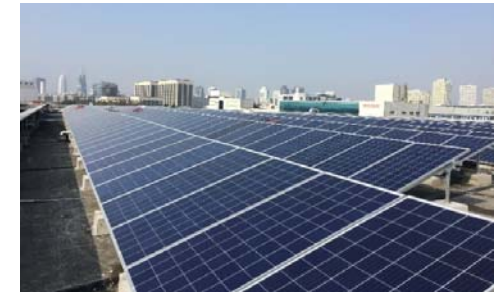
Solar panels at development site in Shanghai
